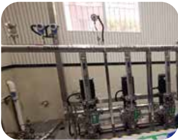
Water quality monitoring of tap water network
