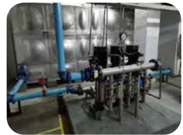
Monitoring of secondary water supply of tap water
